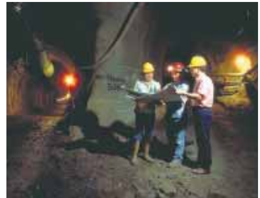
Right: The Exploratory Tunnel saved the State millions by eliminating geological uncertainties.
