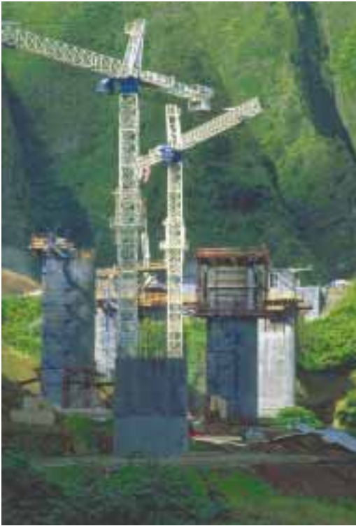
Drilled shafts for cast in place concrete piers were used instead of pile driving for piers.
